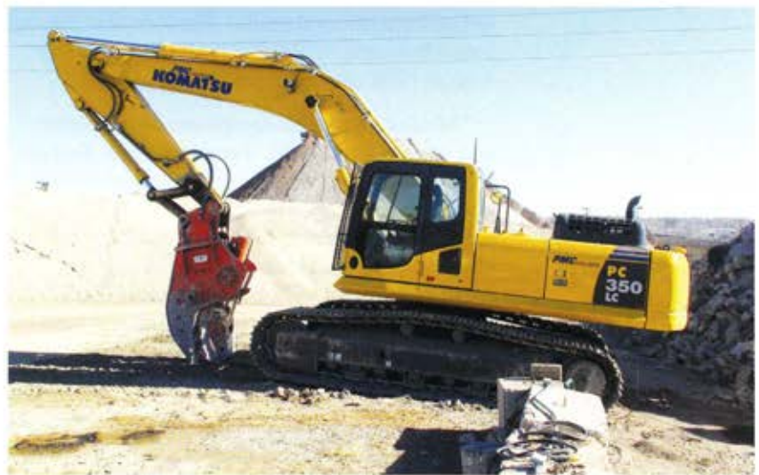
Oxford Recycling uses this Komatsu PC350LC-8 excavator, equipped with an NPK crusher, to pre-size concrete.
